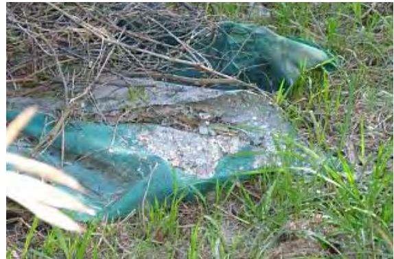
Figure 3 Visible amount of AF on from high-pressure cleaning of an asbestos cement roof.
